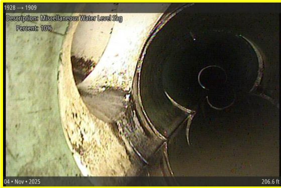
[Grade 2] Miscellaneous Water Level Sag at 206.5 ft
