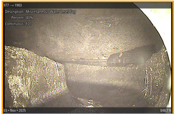
[Grade 3] Miscellaneous Water Level Sag (finish) at 048.7 ft
