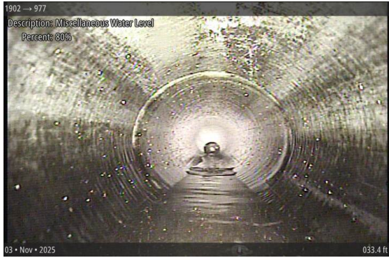
Miscellaneous Water Level at 000.0 ft
