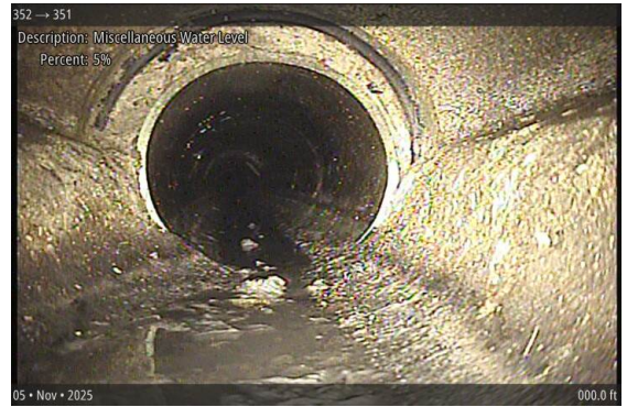
Miscellaneous Water Level at 000.0 ft
