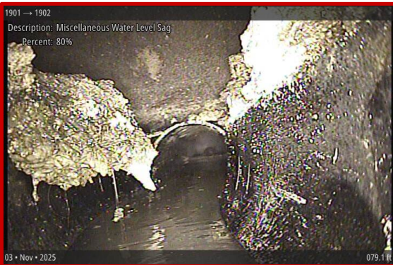
[Grade 5] Miscellaneous Water Level Sag at 079.1 ft
