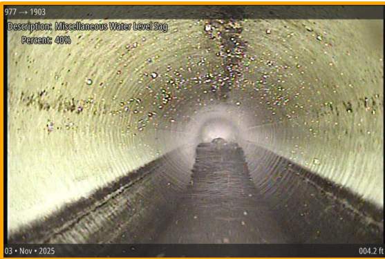
[Grade 3] Miscellaneous Water Level Sag (start) at 000.2 ft
