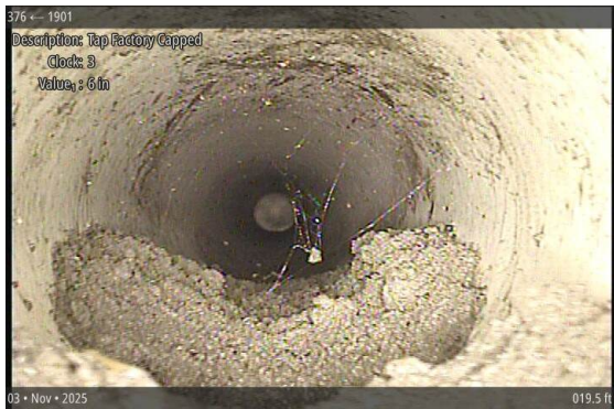
Tap Factory Capped at 019.5 ft, 3 o'clock
