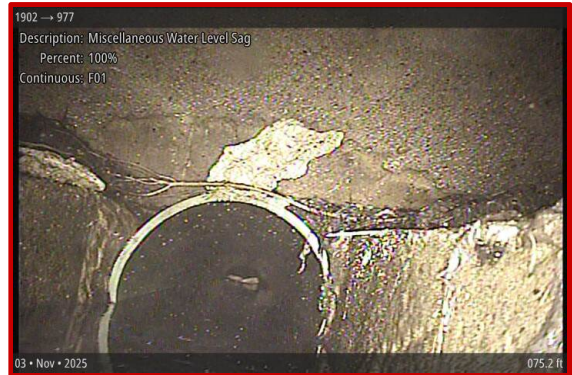
[Grade 5] Miscellaneous Water Level Sag (finish) at 075.1 ft
