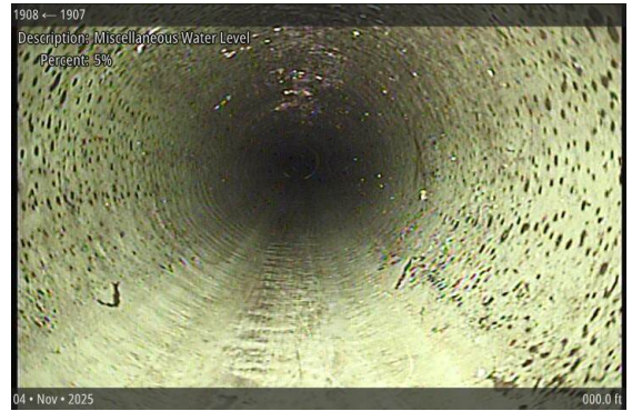
Miscellaneous Water Level at 000.0 ft
