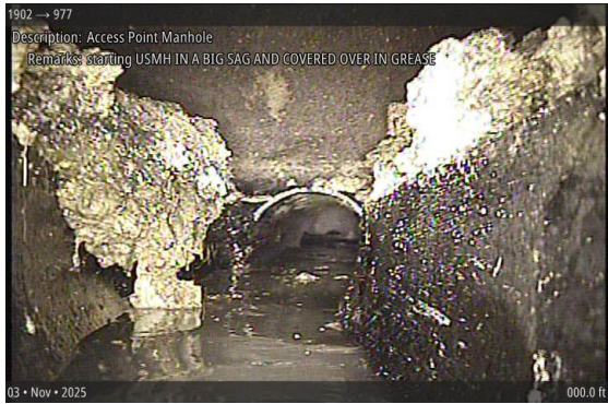
Access Point Manhole at 000.0 ft | starting USMH IN A BIG SAG AND COVERED OVER IN GREASE
