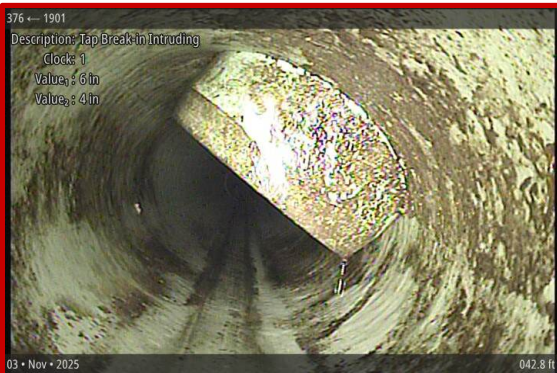
[Grade 5] Tap Break-in Intruding at 042.8 ft, 1 o'clock
