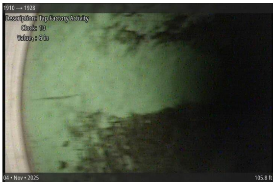
Tap Factory Activity at 105.8 ft, 10 o'clock
