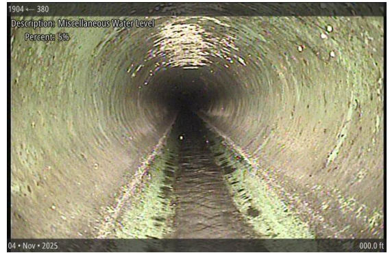
Miscellaneous Water Level at 000.0 ft
