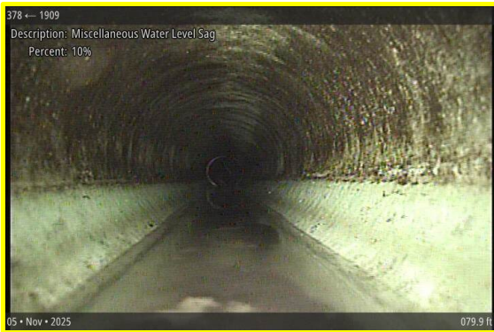
[Grade 2] Miscellaneous Water Level Sag at 079.3 ft
