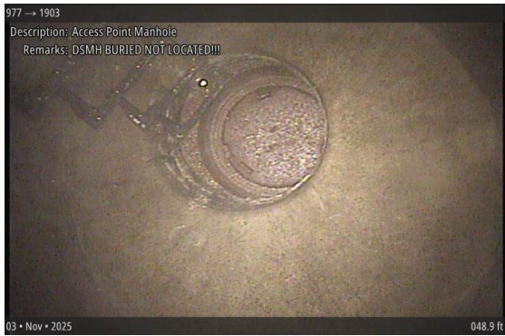
Access Point Manhole at 048.9 ft | DSMH BURIED NOT LOCATED!!!
