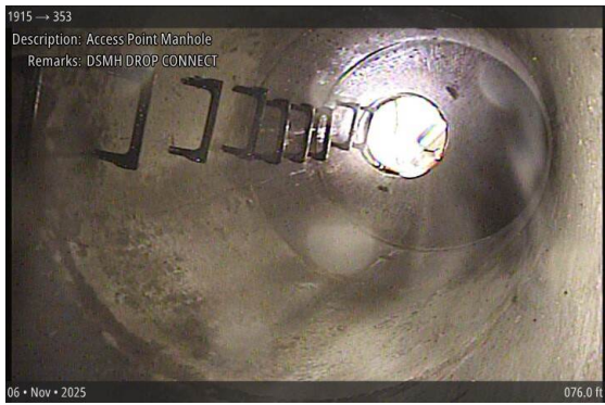
Access Point Manhole at 076.0 ft | DSMH DROP CONNECT
