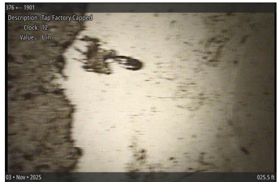
Tap Factory Capped at 025.5 ft, 12 o'clock
