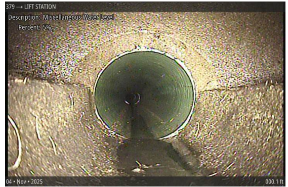
Miscellaneous Water Level at 000.0 ft
