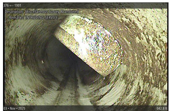
Miscellaneous Survey Abandoned at 042.8 ft | INTRUDING SERVICE
