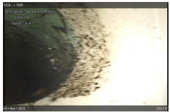
Tap Factory Activity at 214.1 ft, 10 o'clock
