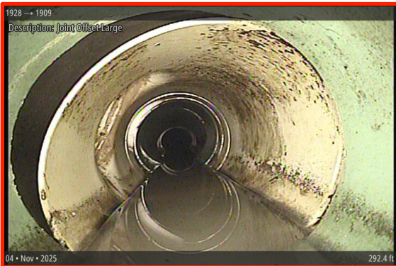
[Grade 4] Joint Offset Large at 292.4 ft
