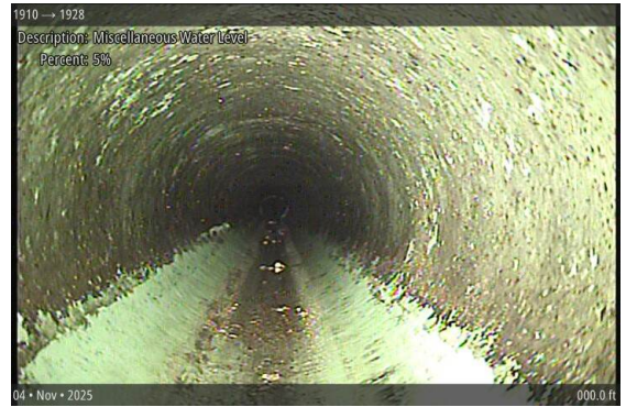
Miscellaneous Water Level at 000.0 ft
