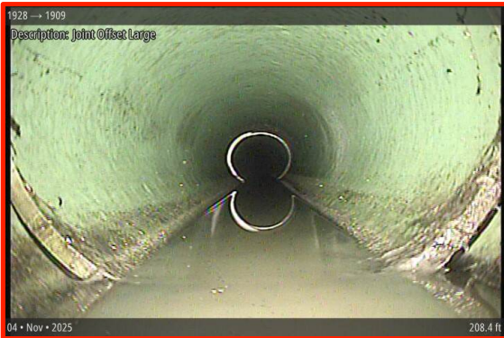
[Grade 4] Joint Offset Large at 208.4 ft
