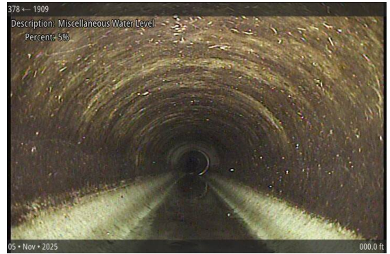
Miscellaneous Water Level at 000.0 ft
