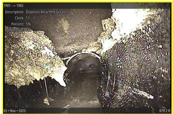
[Grade 2] Deposits Attached Grease (finish) at 079.1 ft, 11 - 1 o'clock
