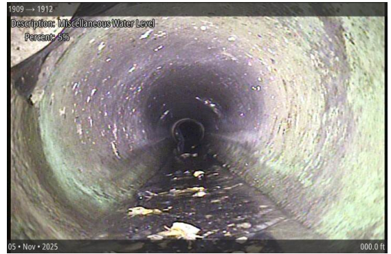
Miscellaneous Water Level at 000.0 ft
