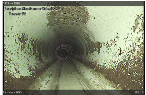
Miscellaneous Water Level at 000.0 ft
