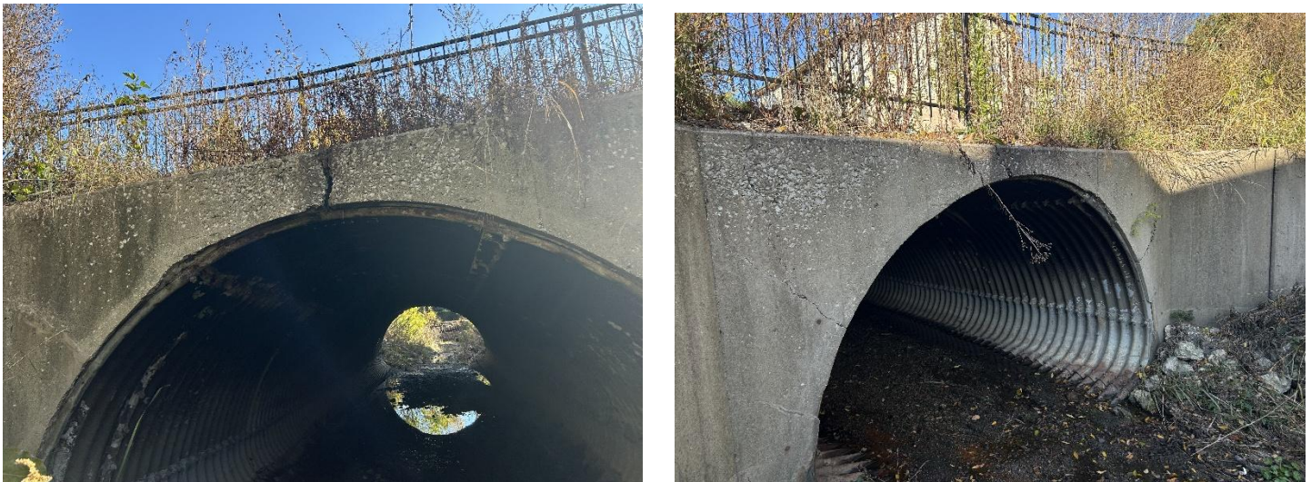
Figure 2: Existing CMP along 49 th Street Ditch at the Creek Drive crossing appears to be in fair condition. Some cracking is visible along the west headwall.
