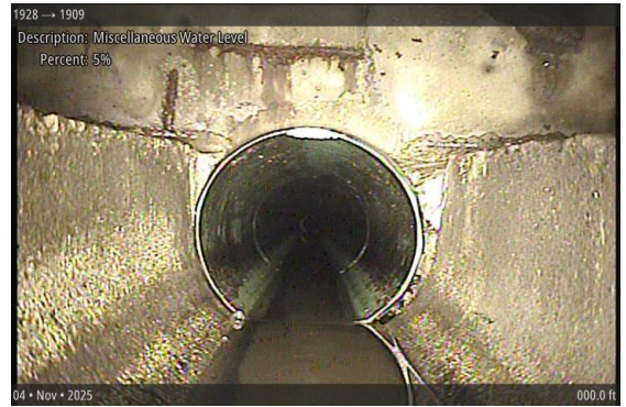
Miscellaneous Water Level at 000.0 ft
