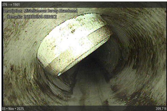
Miscellaneous Survey Abandoned at 209.7 ft | INTRUDING SERVICE
