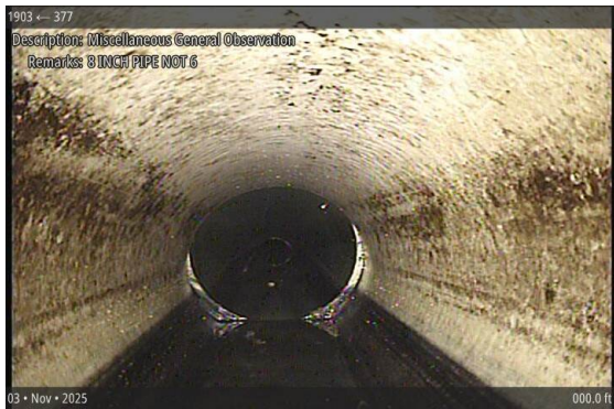
Miscellaneous General Observation at 000.0 ft | 8 INCH PIPE NOT 6
