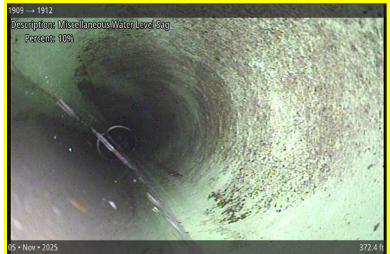
[Grade 2] Miscellaneous Water Level Sag at 372.4 ft
