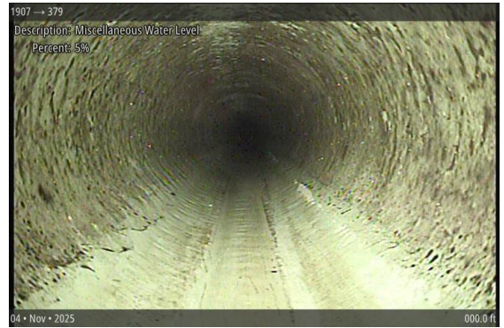
Miscellaneous Water Level at 000.0 ft
