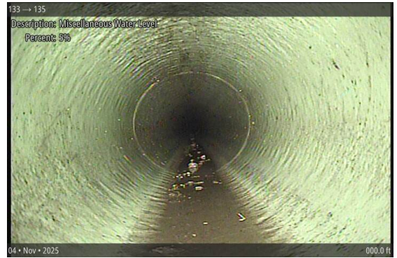
Miscellaneous Water Level at 000.0 ft
