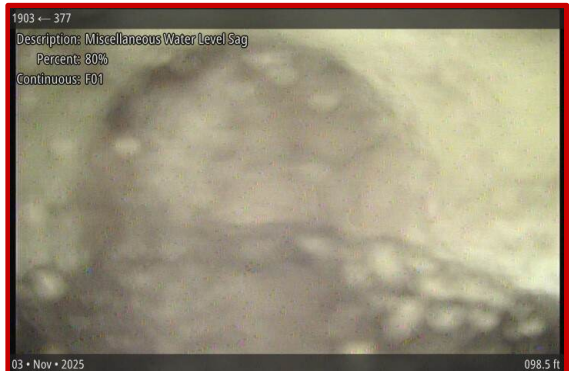
[Grade 5] Miscellaneous Water Level Sag (finish) at 098.5 ft
