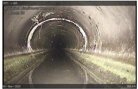
Miscellaneous Water Level at 000.0 ft
