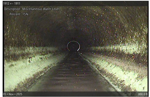
Miscellaneous Water Level at 000.0 ft
