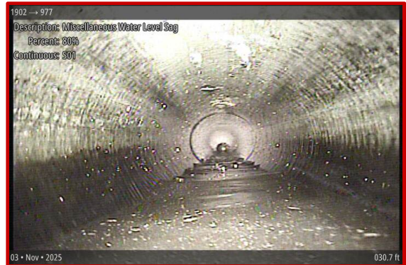
[Grade 5] Miscellaneous Water Level Sag (start) at 000.1 ft
