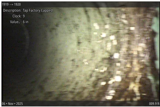
Tap Factory Capped at 009.9 ft, 9 o'clock
