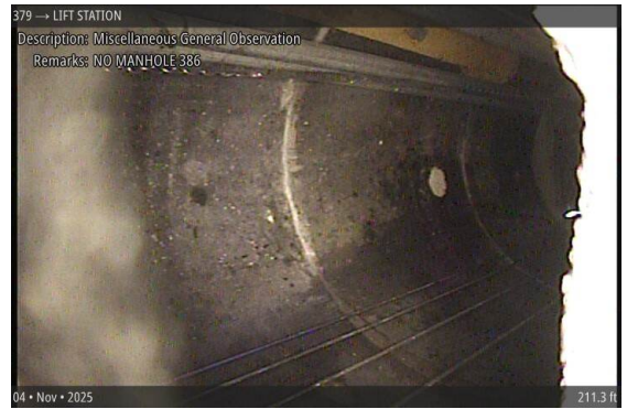
Miscellaneous General Observation at 211.3 ft | NO MANHOLE 386
