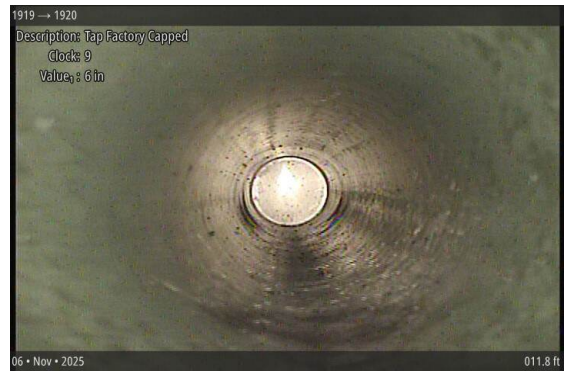
Tap Factory Capped at 011.8 ft, 9 o'clock
