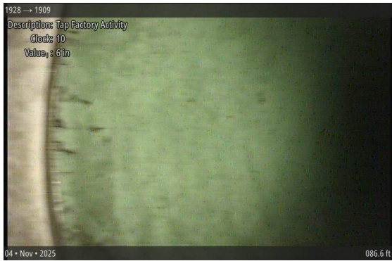
Tap Factory Activity at 086.6 ft, 10 o'clock
