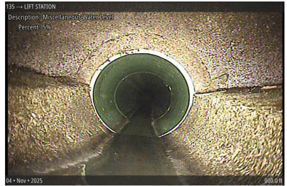
Miscellaneous Water Level at 000.0 ft
