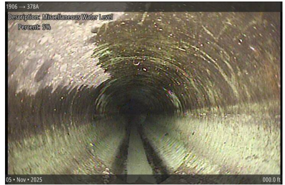
Miscellaneous Water Level at 000.0 ft
