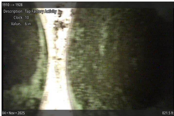
Tap Factory Activity at 021.5 ft, 10 o'clock
