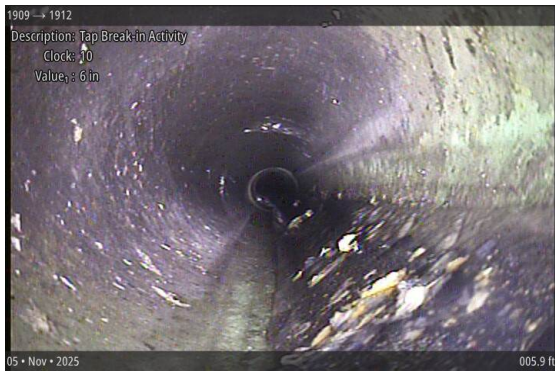
Tap Break-in Activity at 005.9 ft, 10 o'clock
