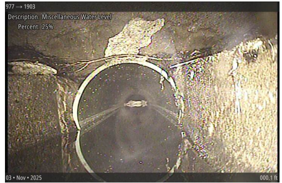
Miscellaneous Water Level at 000.0 ft
