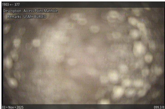
Access Point Manhole at 099.3 ft | USMH BURIED
