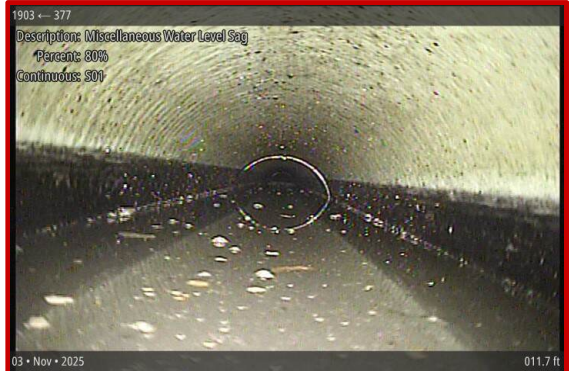
[Grade 5] Miscellaneous Water Level Sag (start) at 011.7 ft
