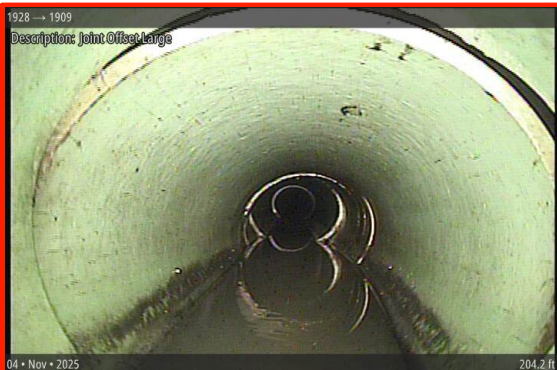
[Grade 4] Joint Offset Large at 204.2 ft
