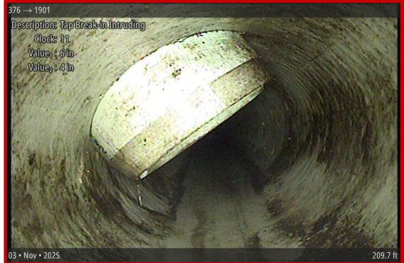
[Grade 5] Tap Break-in Intruding at 209.7 ft, 11 o'clock
