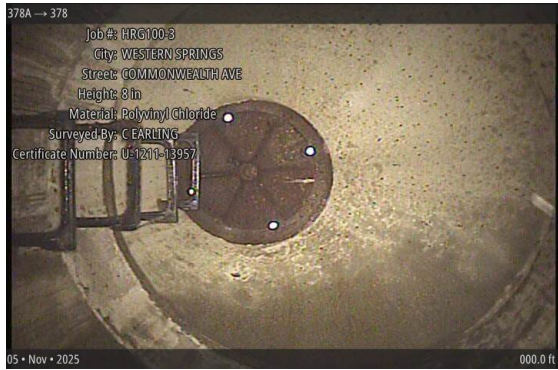
Miscellaneous Water Level at 000.0 ft
