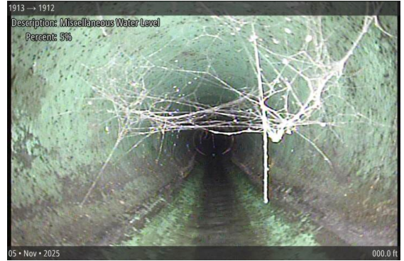
Miscellaneous Water Level at 000.0 ft
