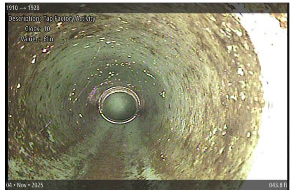
Tap Factory Activity at 043.8 ft, 10 o'clock
