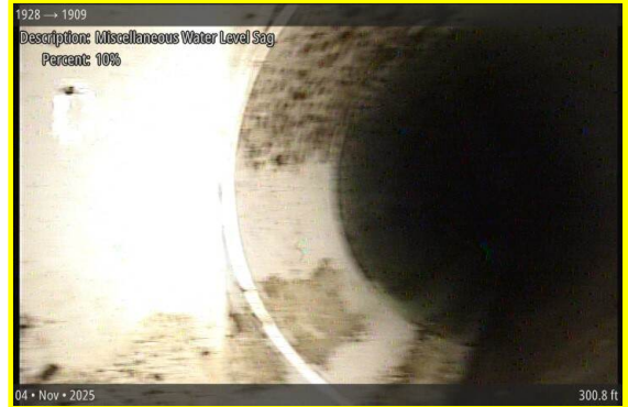
[Grade 2] Miscellaneous Water Level Sag at 300.8 ft
