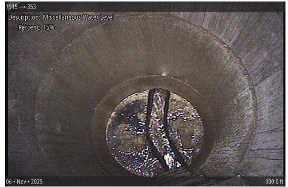
Miscellaneous Water Level at 000.0 ft
