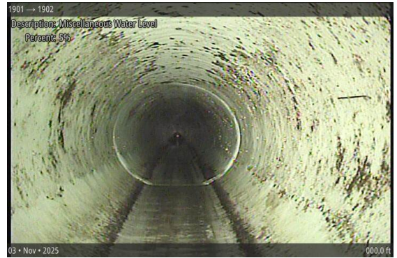
Miscellaneous Water Level at 000.0 ft
