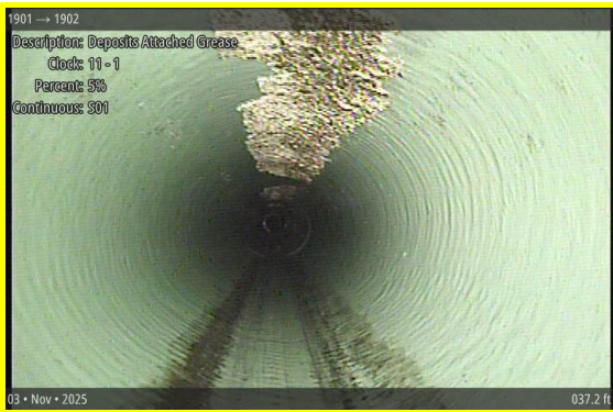
[Grade 2] Deposits Attached Grease (start) at 037.2 ft, 11 - 1 o'clock
