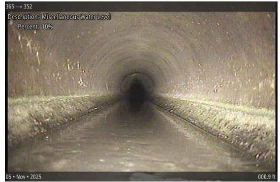
Miscellaneous Water Level at 000.0 ft
