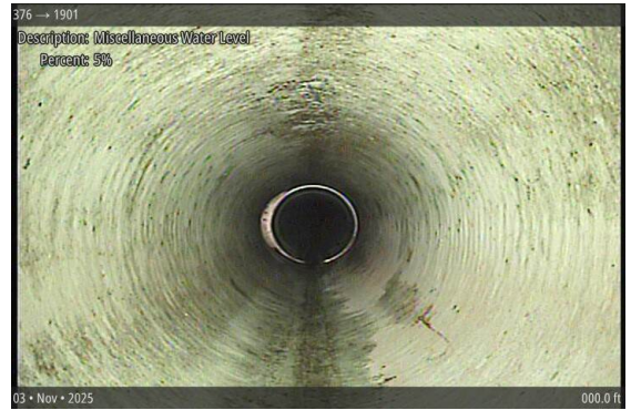
Miscellaneous Water Level at 000.0 ft
