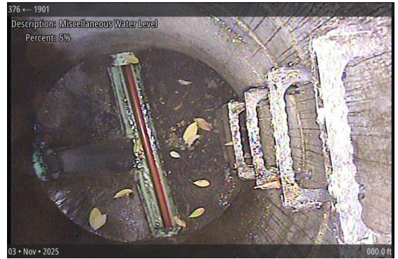
Miscellaneous Water Level at 000.0 ft
