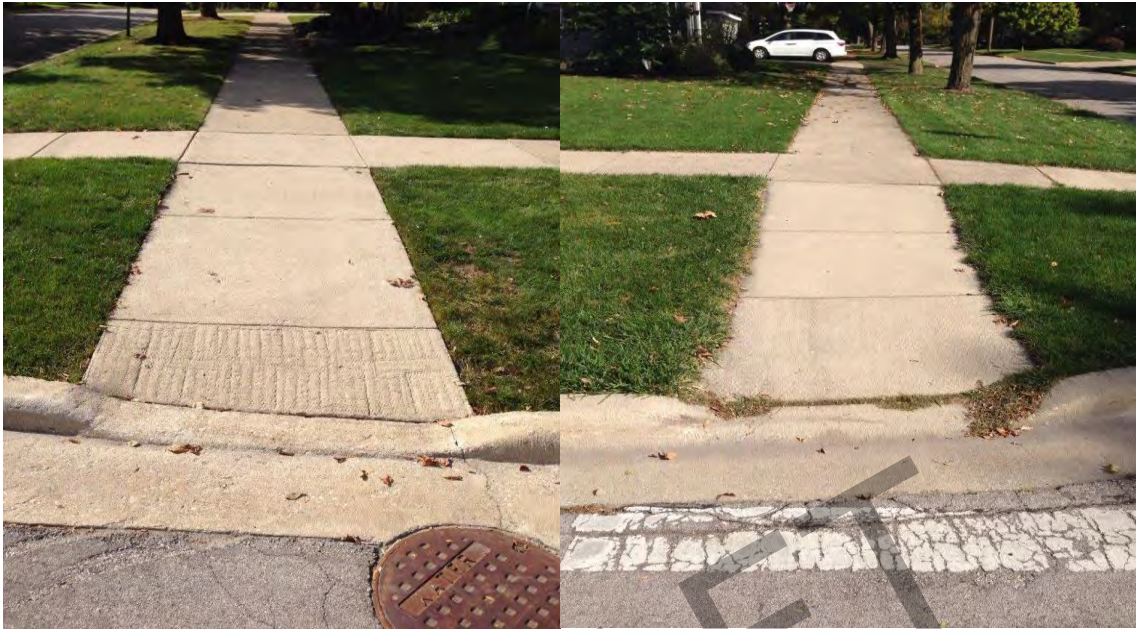
The above examples show crosswalks that are non-compliant with both previous and current ADA Standards.
