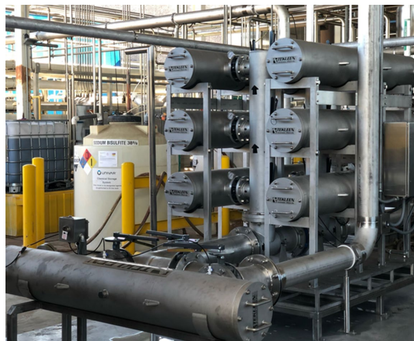
Figure 5 Typical Configuration Stacked Filters (Tekleen, Arizona)
